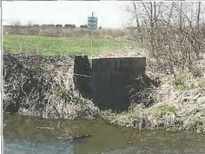
Photo 15 – CSO 004 outfall into Cedar Creek. Located just east of the equalization basin at the Lowell Treatment Plant. Note: No evidence of solids build up or floatable materials.
