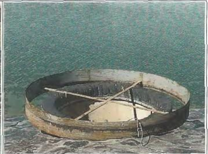
Photo 14 – Close-up view of CSO 004 overflow pipe from equalization basin. Scum baffle provides for floatable control.
