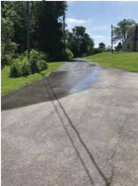
completed "repair" after water main fixed
