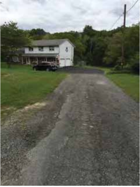
Erosion from water main break on Betty's private lane. The town did not fix this. We paid to have rocks fill in the ruts.
